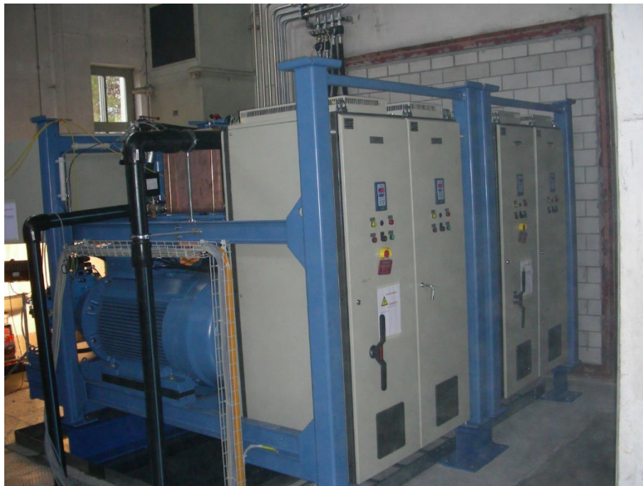
Figure 11 – Hydraulic power station with four independent pumps delivering up to 250 kW each.
