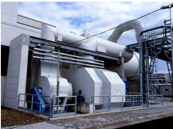
Fig 13: Fans and pipes of the EFS system.
