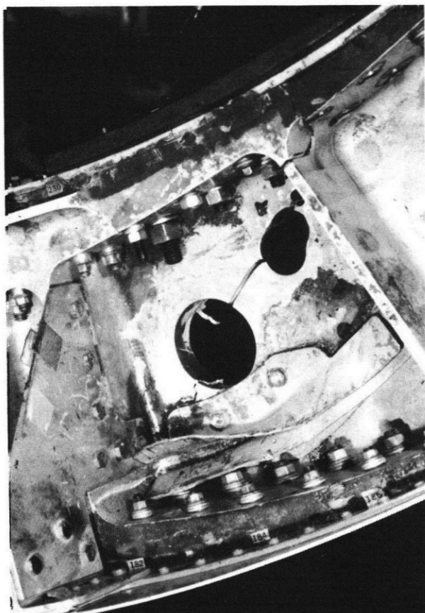
Figure 17. Final failure at the fuel pipe holes
